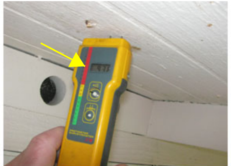
93% moisture reading in eve
