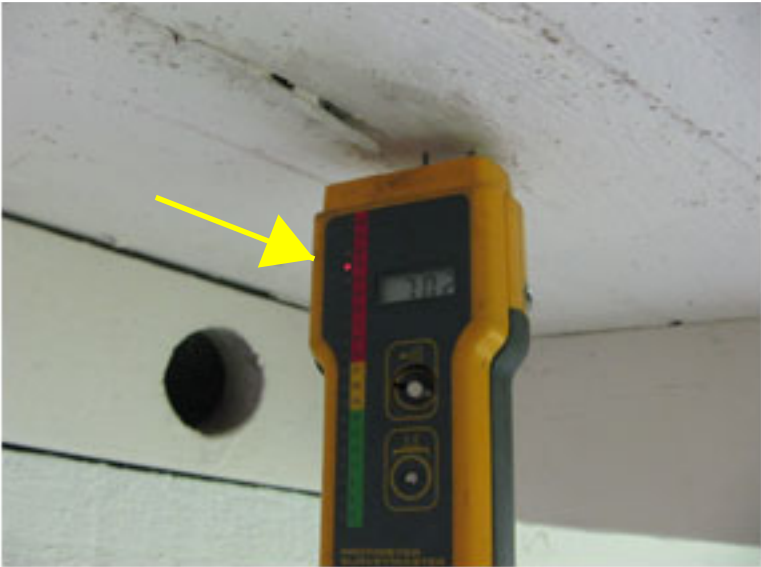
70% moisture reading in eve
