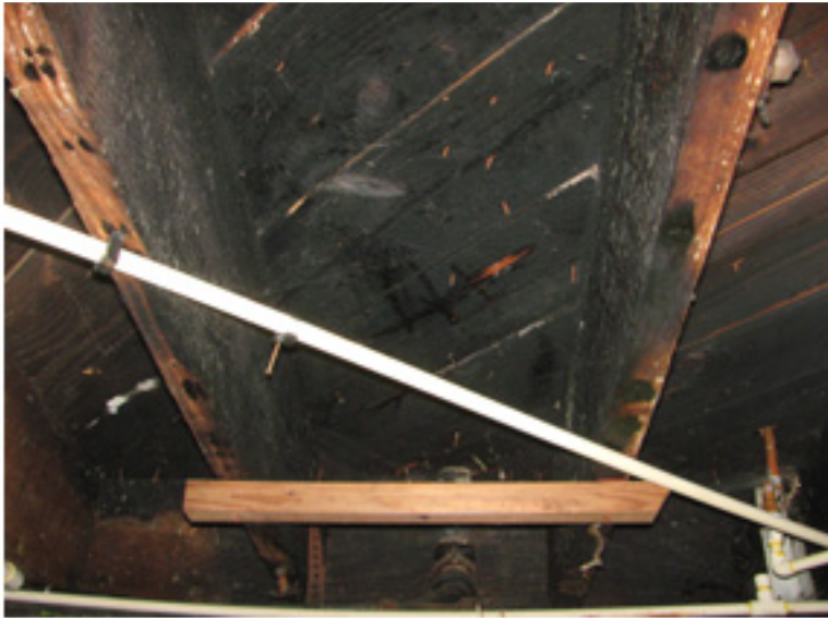
Signs of a past fire in the basement
