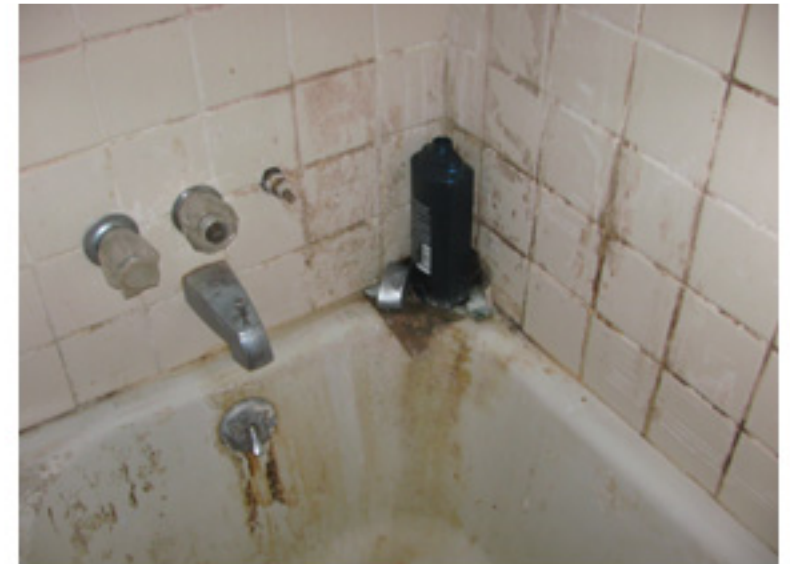
Main bathroom has poor tile repair work
