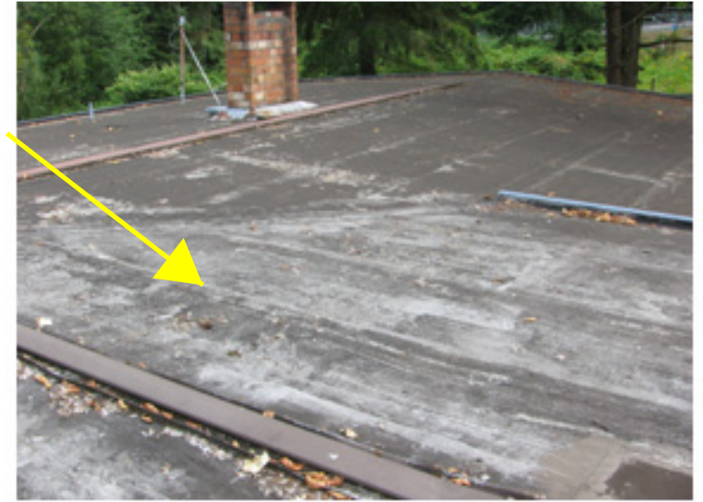
Roof is at the end of its useful life
