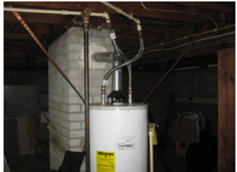
Hot water tank is poorly strapped
