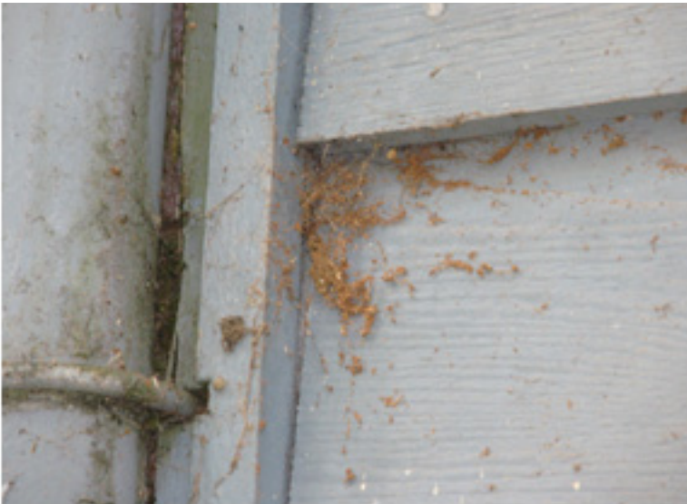
Signs of pest activity below the weatherhead
