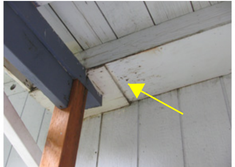
Rot in eave soffit
