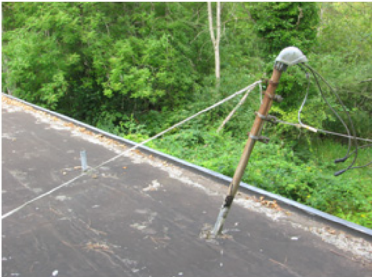
Weather head is bent and not well supported
