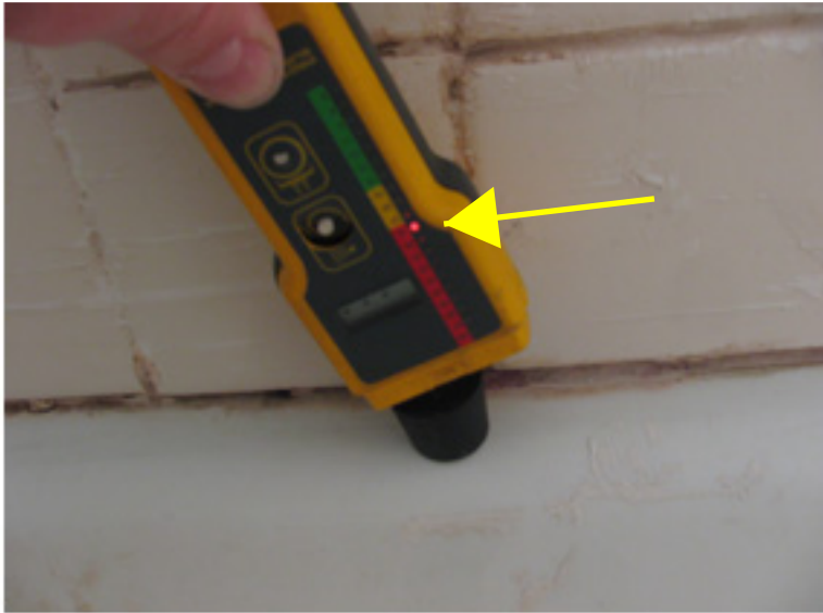
High moisture reading in the main bathroom
