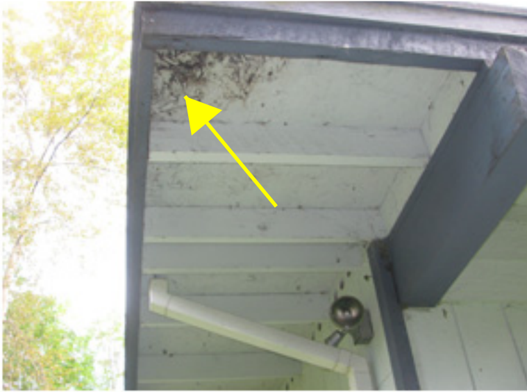
Rot in eaves
