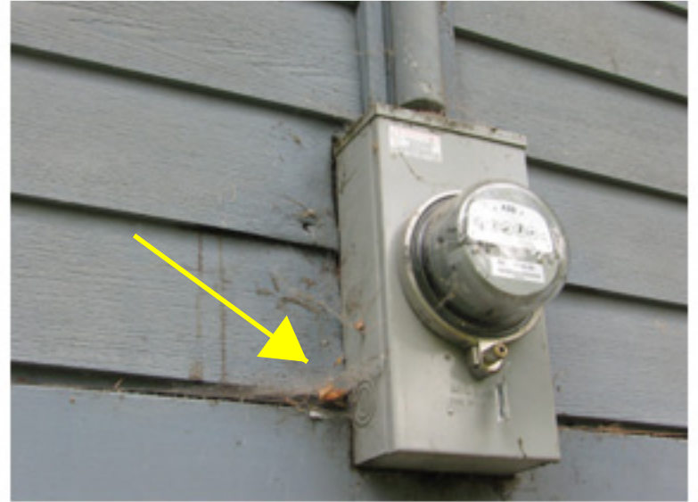
Water damage to siding
