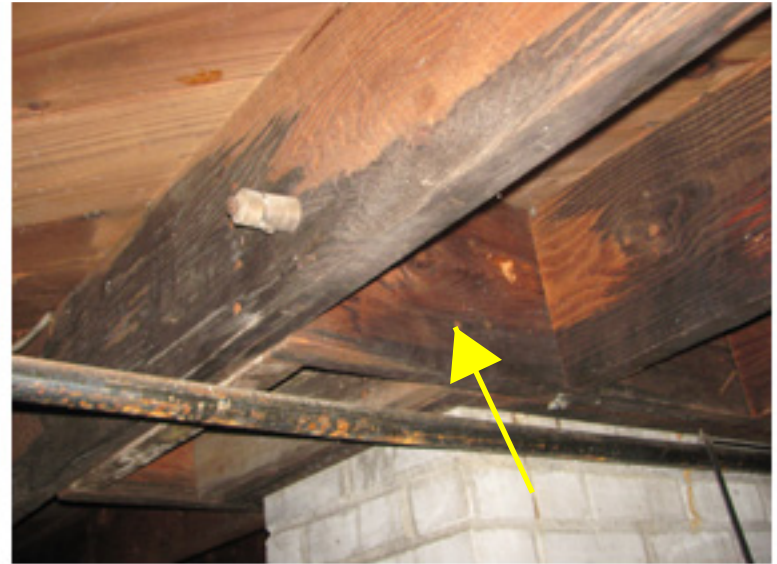
Signs darkening and rot on sub the floor
