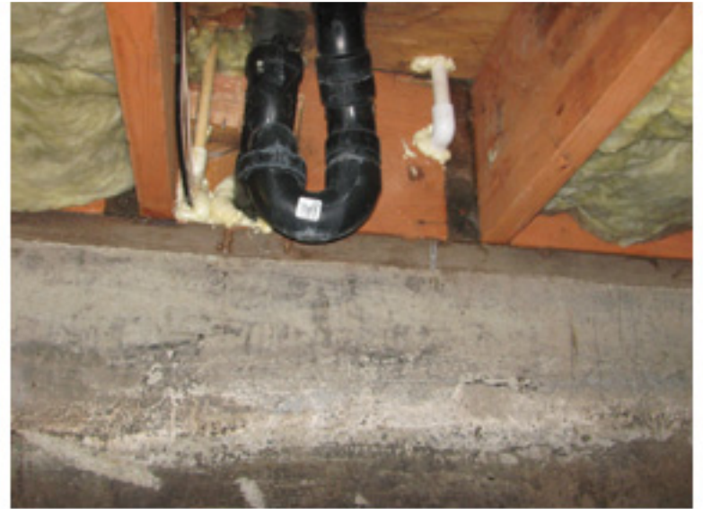
Leak under the master shower
