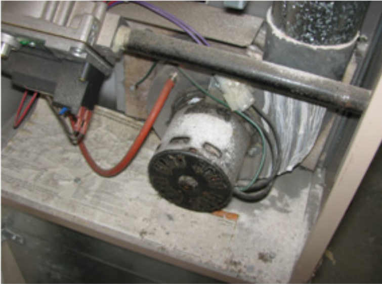
Furnace is very dirty
