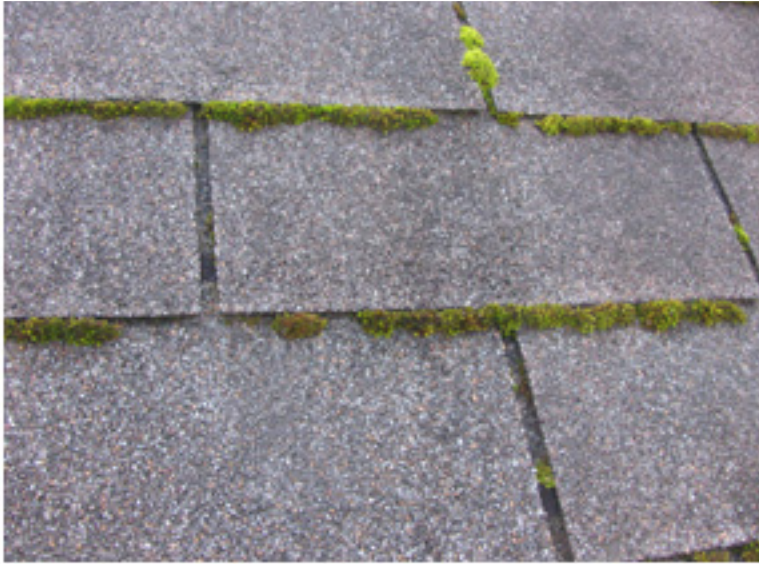
Clean moss off of roof
