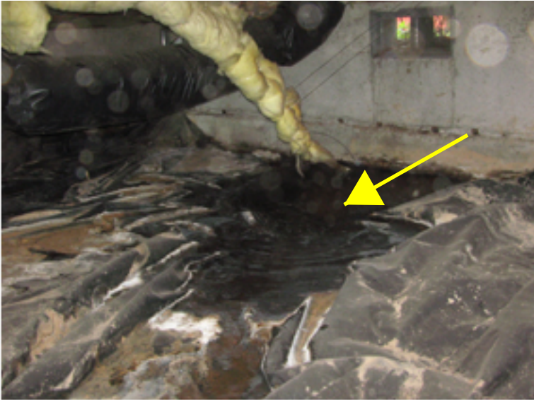
Standing water in the east crawlspace
