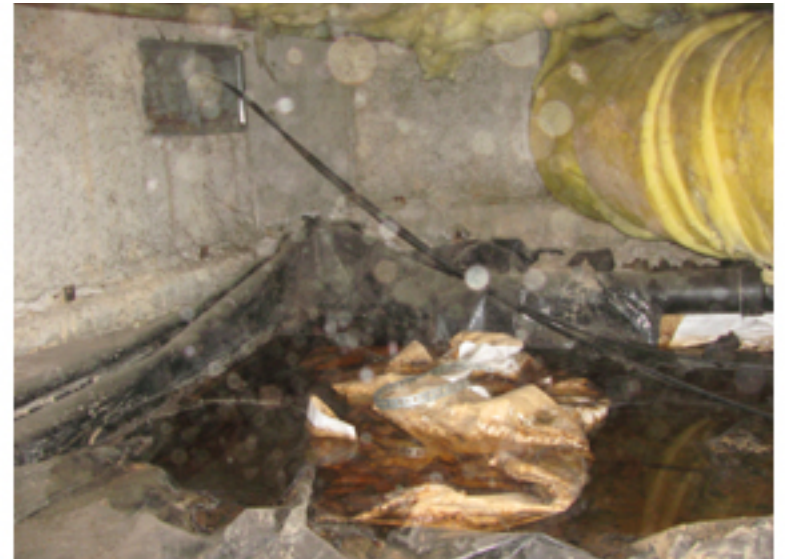
Standing water in the SW corner
