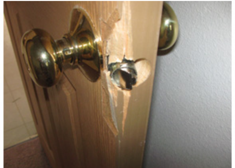
Master bedroom door is damaged
