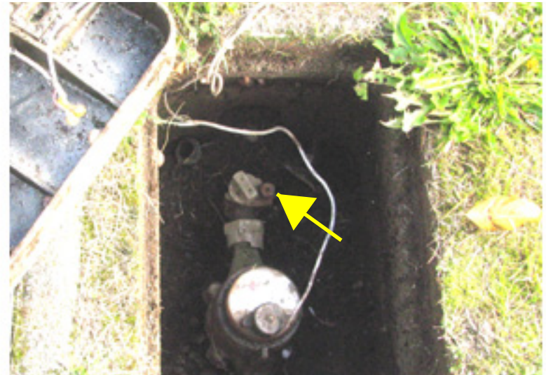
Water service is locked out
