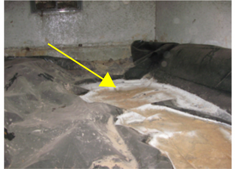
Many water stains on vapor barrier in the crawlspace
