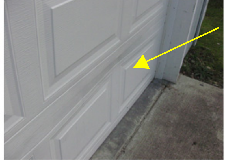
Dent in garage door
