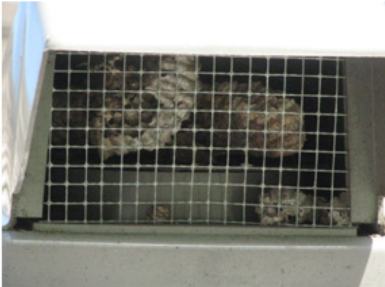
Bees nests in bathroom vent termination hood (on roof)
