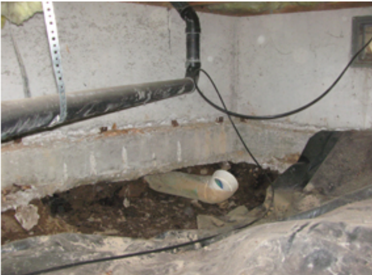
The soil is undermined under the foundation footing (NW corner)
