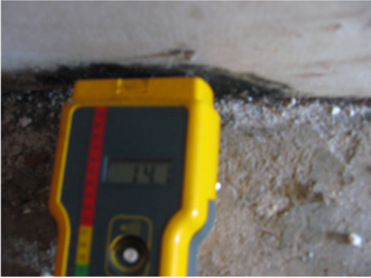
High moisture reading and dark spot on garage wall
