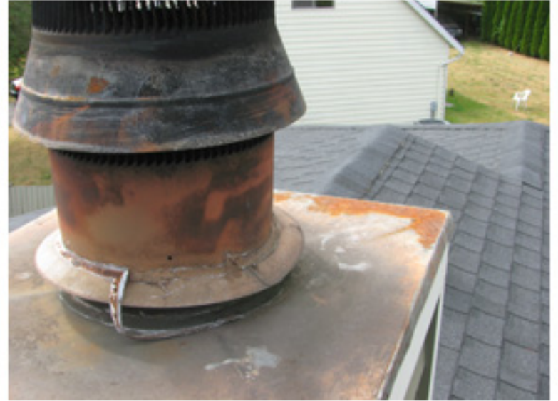
Chimney stack and crown are rusted
