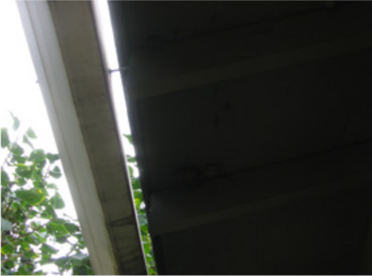
Gutters are separating from house
