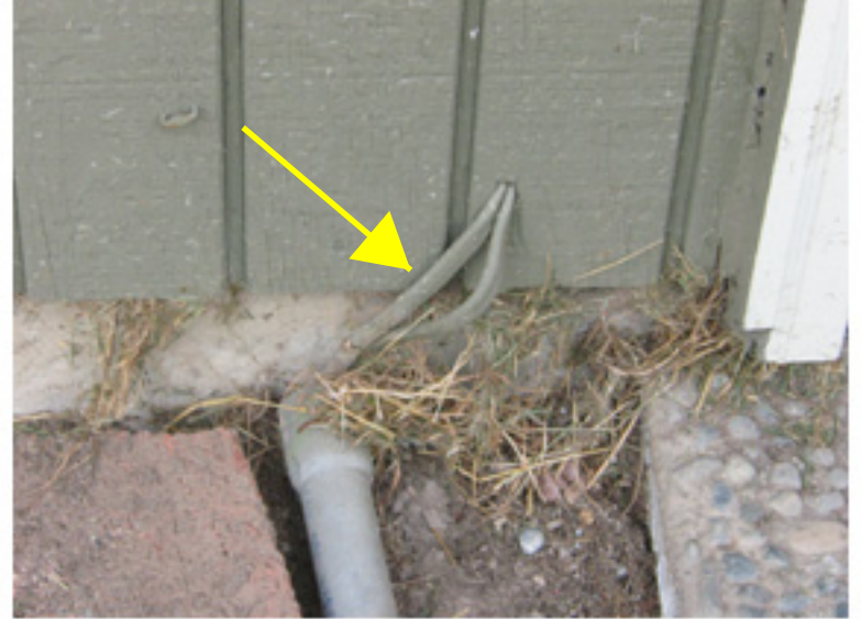
Exposed wires on the exterior
