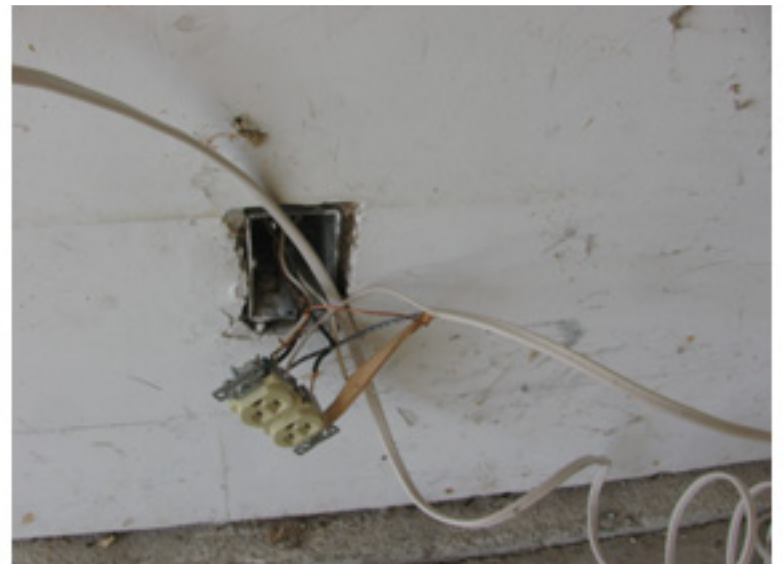
Makeshift wiring in the garage
