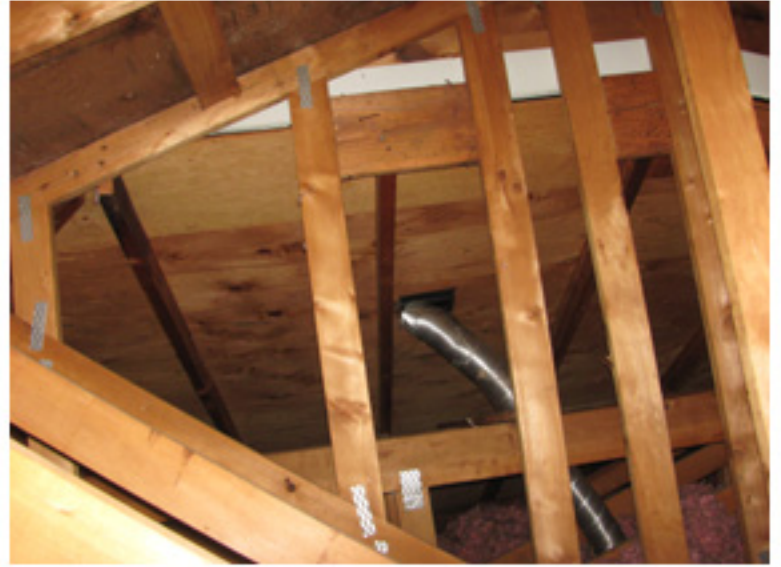
Bathroom vent terminates into attic
