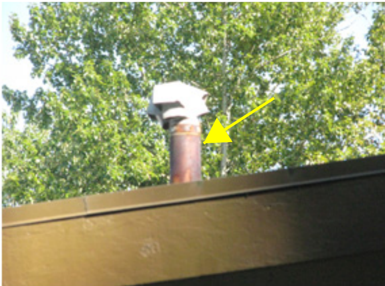
Gas appliance vent stacks are rusted and need replacing
