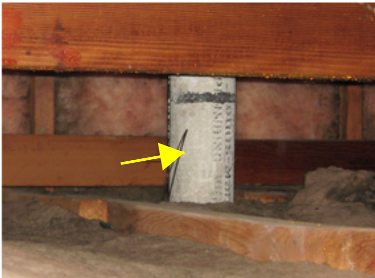
Asbestos lined furnace vent stack in attic
