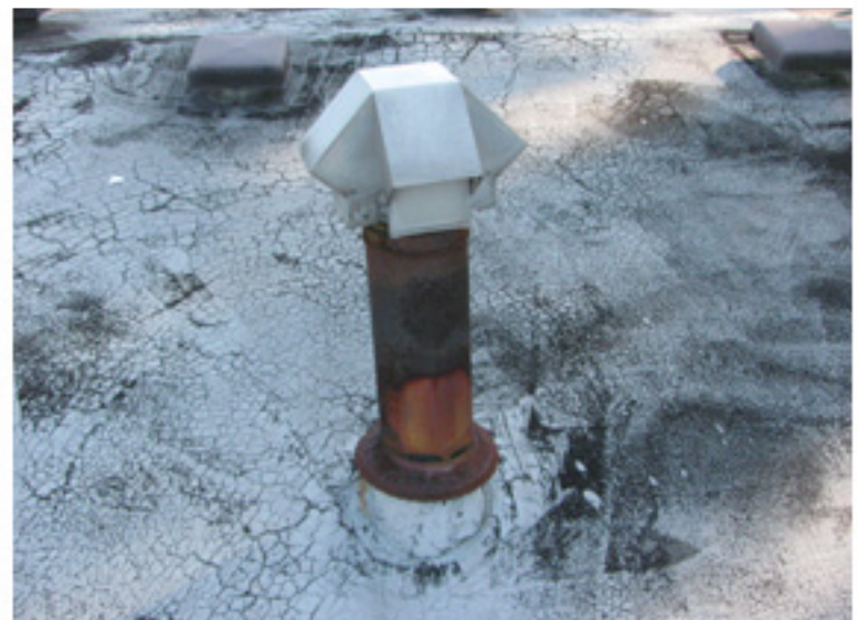
Gas Rusted furnace vent stack
