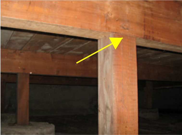
Beam to post junctions need gussets
