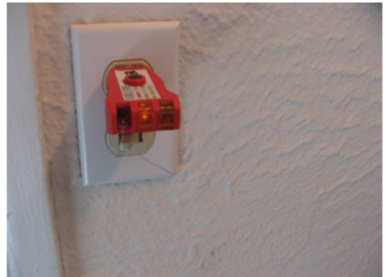
Non-grounded 3-prong outlet in the bathroom
