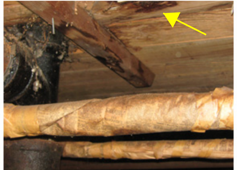
Rot on bathroom sub floor (toilet - shower area)
