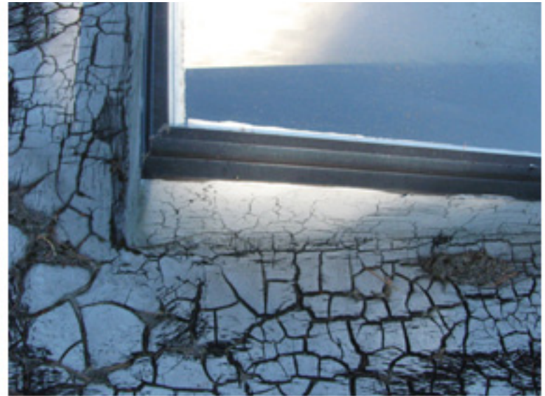
Significant alligatoring on roof
