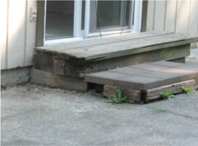
Back patio landing is rotted
