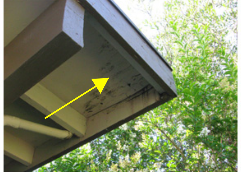
Rot in soffit
