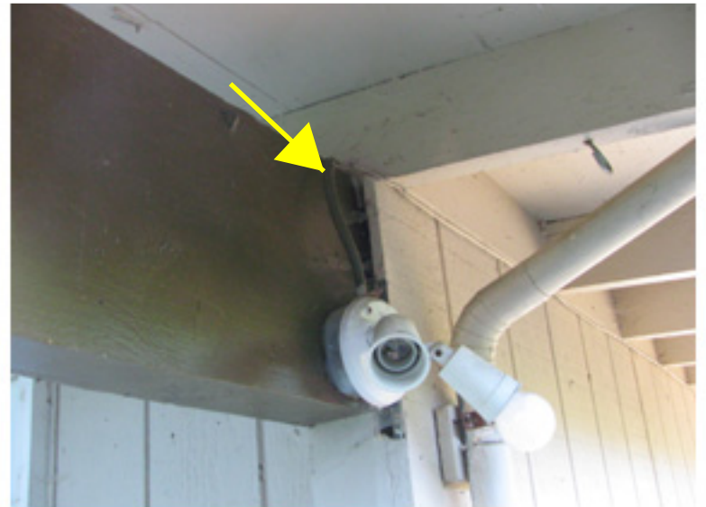
Exposed Romex type wiring on exterior
