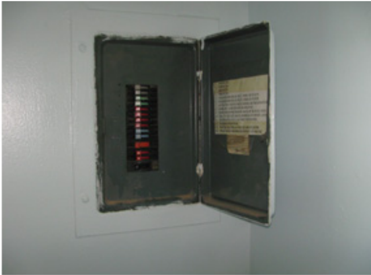
Defective Zinsco brans electric service panel
