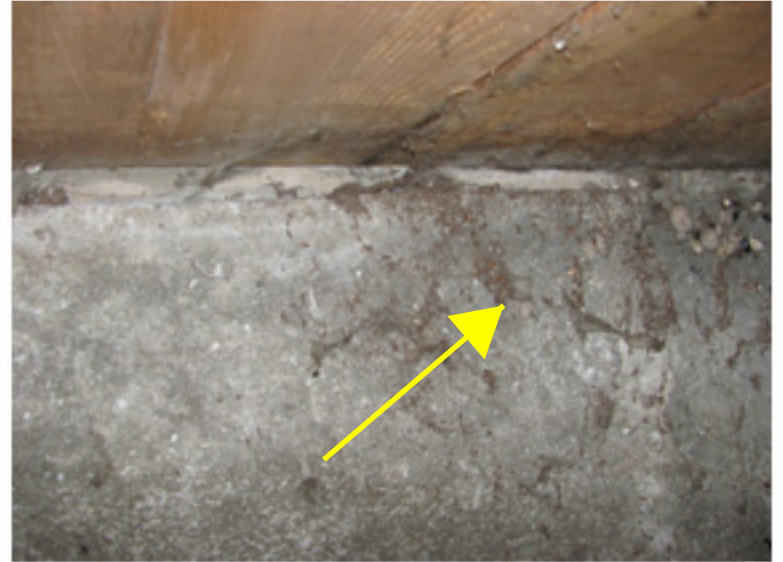
Signs of pest activity in the crawlspace
