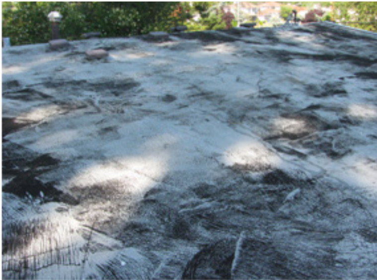
Silver coating is worn out on roof (roof at the end of useful life)
