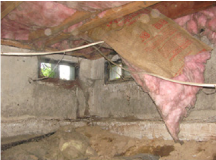
Hang loose wires in the crawlspace
