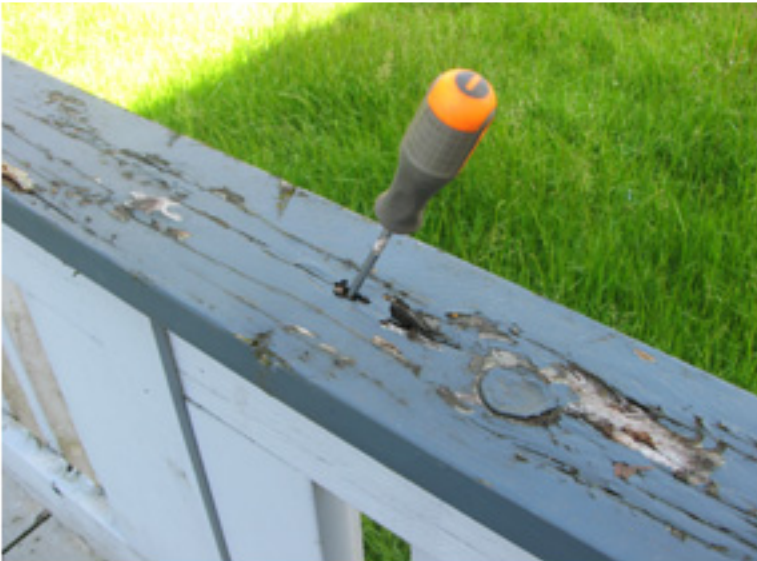
Rot in deck handrail
