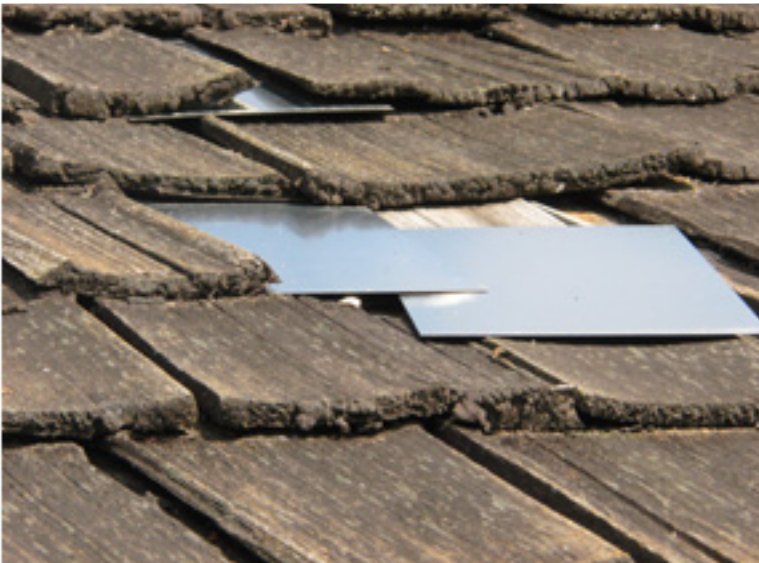
Some shingles are missing
