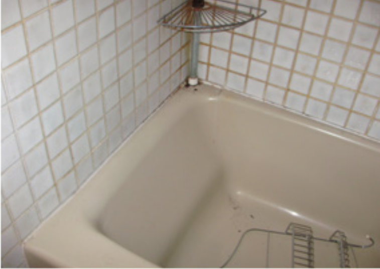
Master bathroom tile needs to be re-grouted and may have damage to wall
