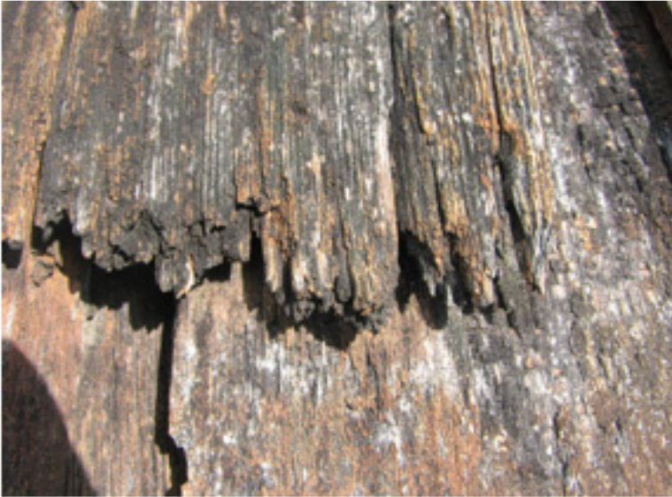
Wood rot in roof shingles
