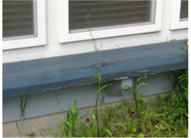
I recommend removing or painting plant shelves
