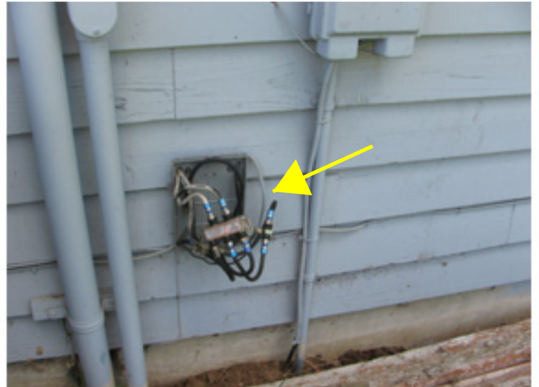
New cable TV junction box cover needed
