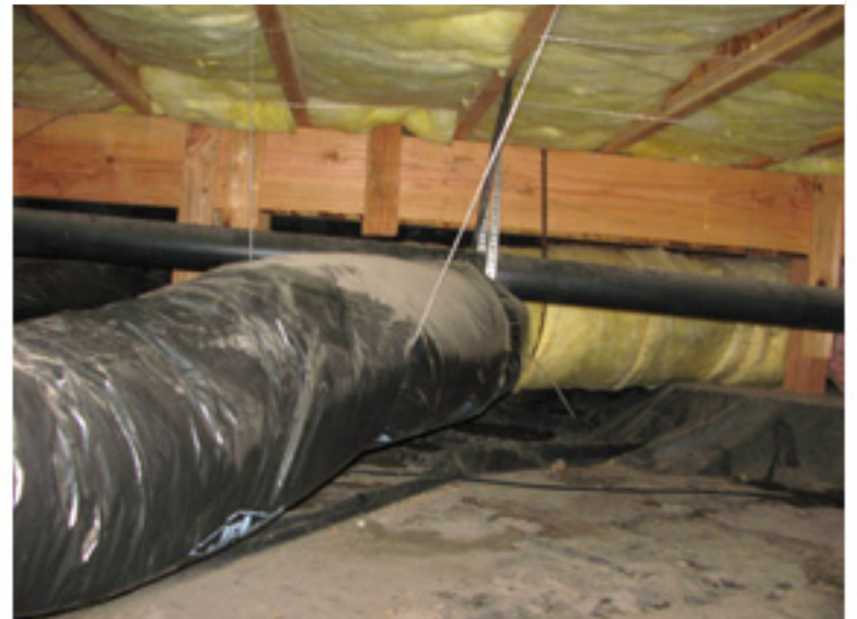
Heat ducts are raised of the ground in the crawlspace
