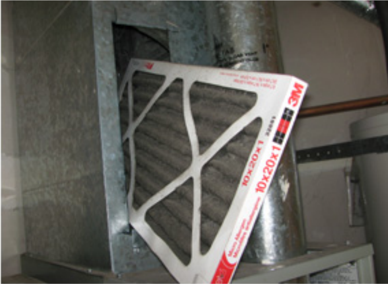
Furnace filters need to be replaced
