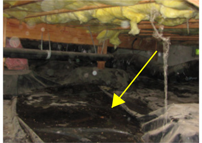
Moisture on top of vapor barrier in the crawlspace
