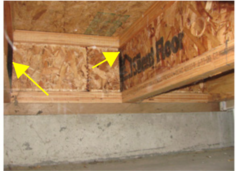
Gaps between joist blocking on garage cantilever
