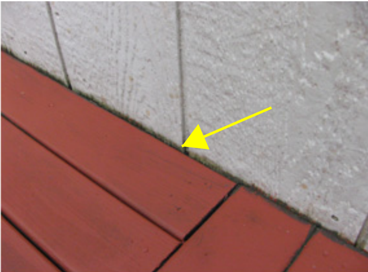
I recommend flashing on deck to wall junction
