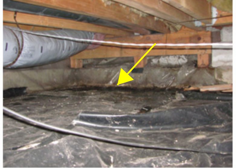
Water under the vapor barrier in the crawlspace
