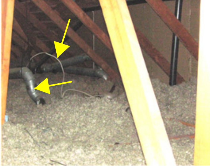
Bathroom vent ducts should terminate through roof
