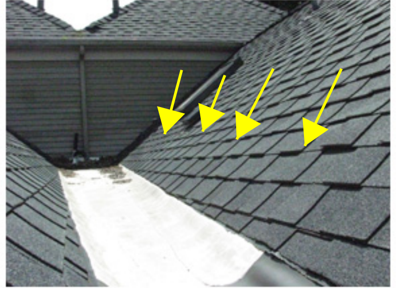
Lower roof vents needed in rafter bays
