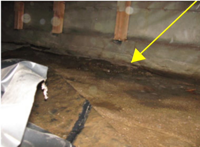
Standing water in the crawlspace
