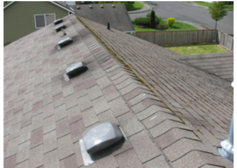
Moss on north side. No moss on south roof.
