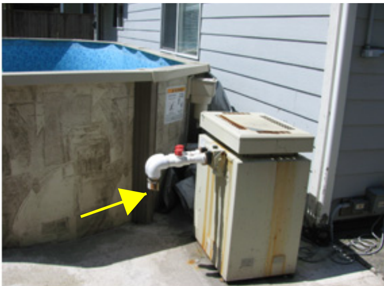
Mechanical to pool has been disconnected
