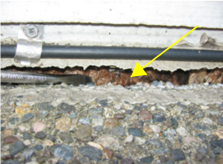
Rot by the front porch
