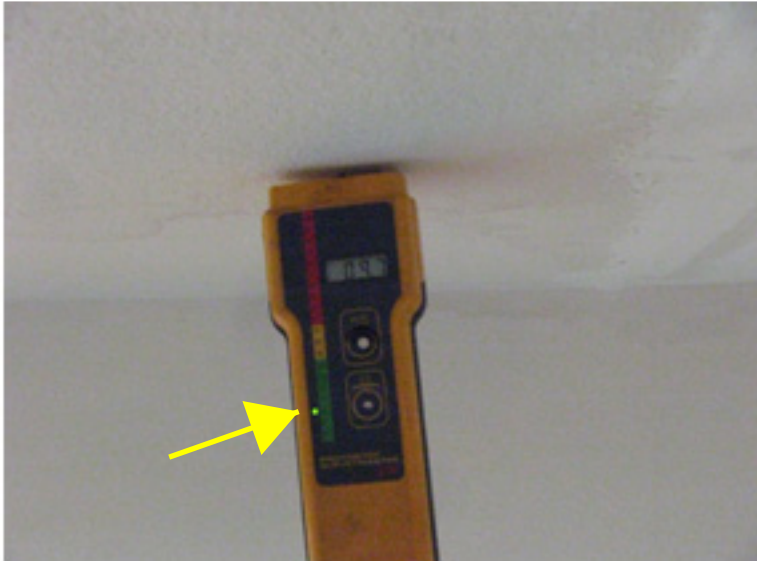
Dry reading on ceiling stain
