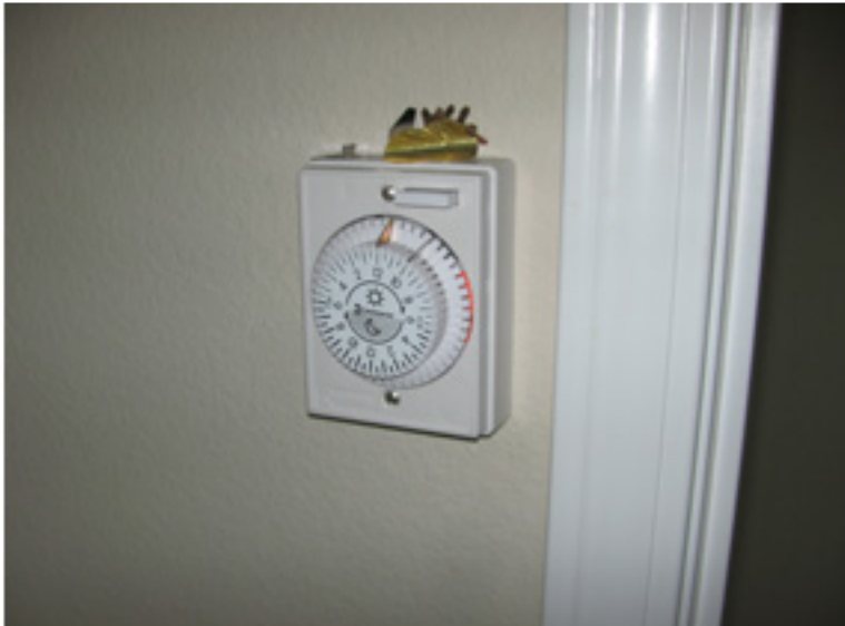
Hole house timer in the laundry room
