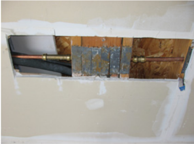
I recommend a sheetrock patch on plumbing repair
