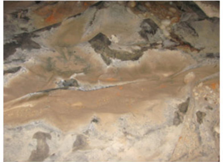
Past water stains on vapor
