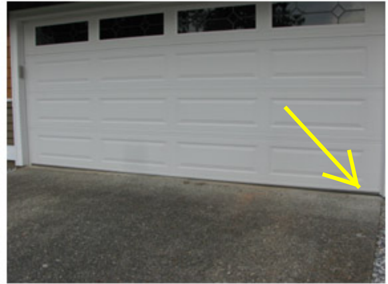
Garage slab has settled
