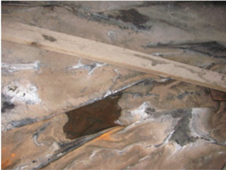
Small amount of water on vapor of vapor barrier
