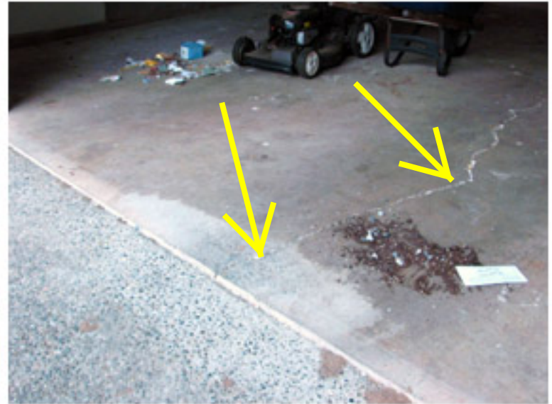
Garage slab crack and grinded
