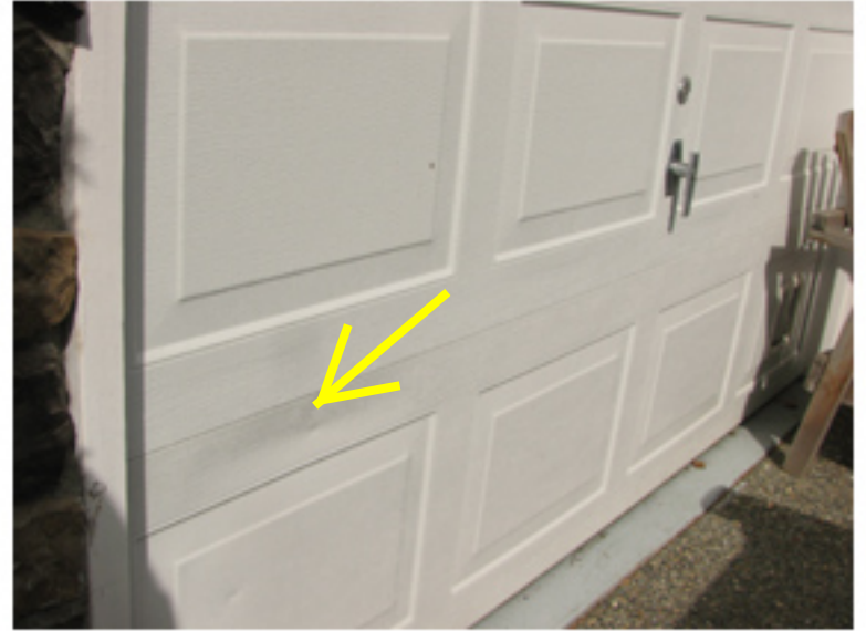
Small dent in garage door
