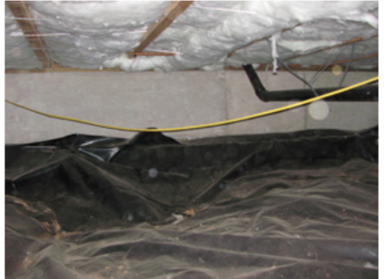
Hang wire that is low in crawlspace
