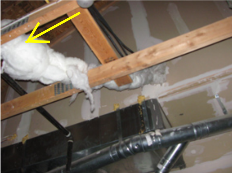
Hose bibb supply pipe running in garage
